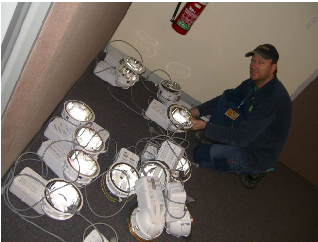
Image: Changeover fittings at Victoria University.
